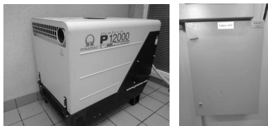
Fig. 2. Generator ProTech P12000 and ATG system
